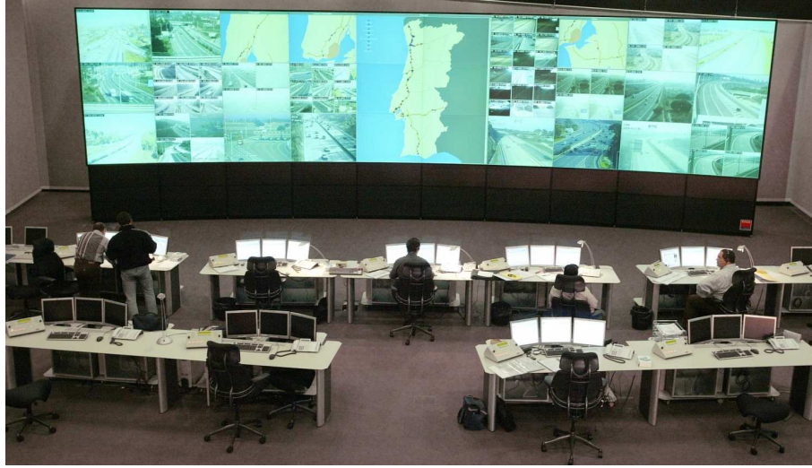
Figure 1.1: Traffic Control Center at Carcavelos, Portugal. The surveillance of the highways operated by Brisa all over the country is performed in this Traffic Control Center.
